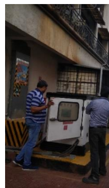
Fiber Cables leading upto the Equipment
