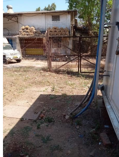
Fiber Cables leading upto the Equipment
