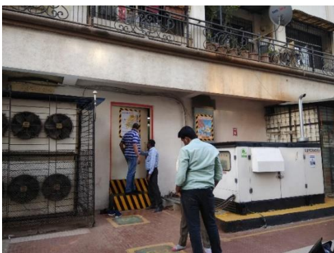
Equipment Location, Kalyan
