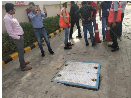
Delhi Fibers Duct at the Equipment Location
