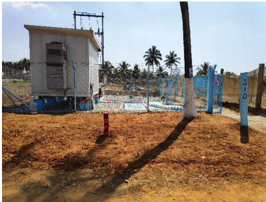
Equipment Location, Whitefield, Bengaluru
